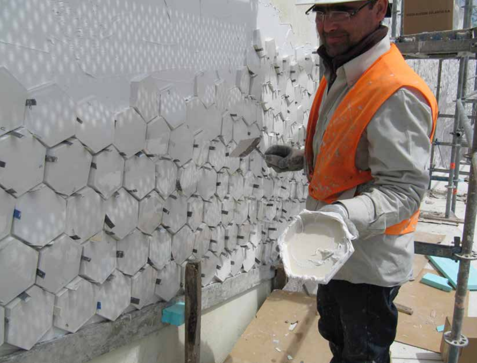
Because of uneasy access on vertical surfaces, installers could cover only 5 m 2 per day per person.
