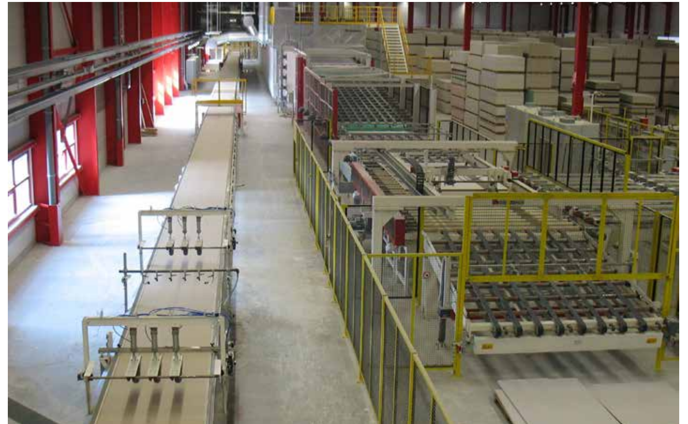
Saving energy, reducing CO 2 emissions and achieving a sustainable bottom line in terms of production are ever-present topics that are also gaining importance in the gypsum industry.
