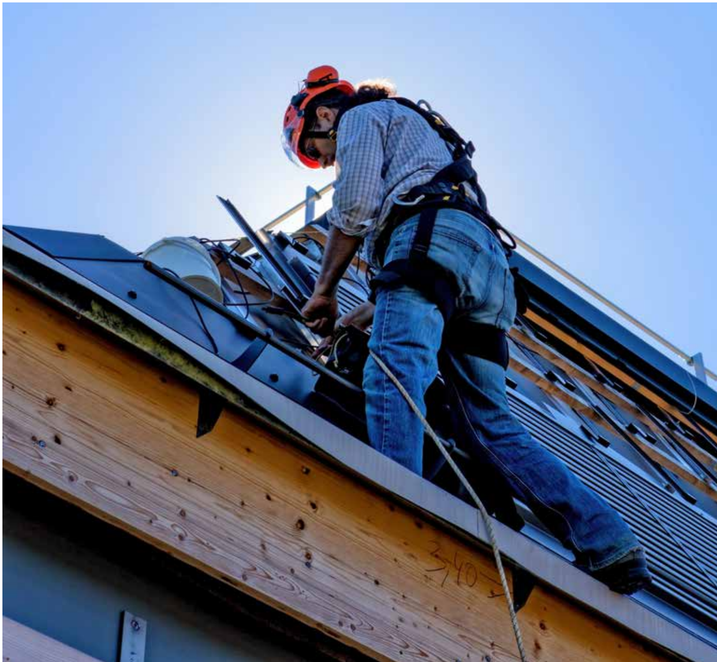
The sloped metal roof is waterproofed by Sarnafil® TG66-15 membrane system including 2 layers of mineral wool thermal insulation.
