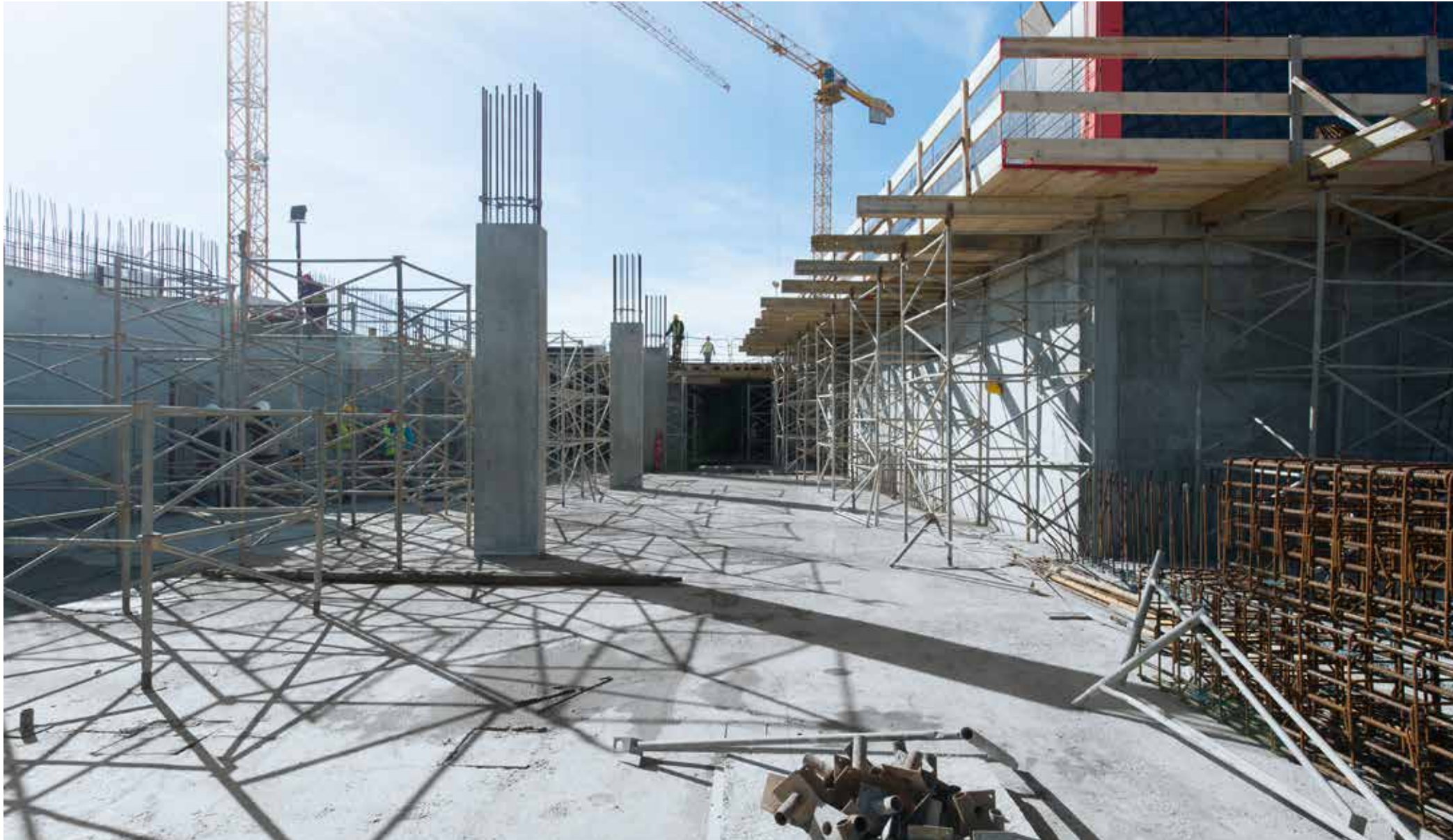
The nearby river creates special challenges for the waterproofing concept for the building foundations. Although the theater site has been raised to a level five meters above the river, some parts of the building are still permanently below the water level. Hence there are exceptionally high requirements for reliable waterproofing systems.
